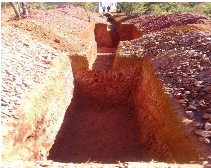
Construction of this septic and soak way tanks is an urgent need.
